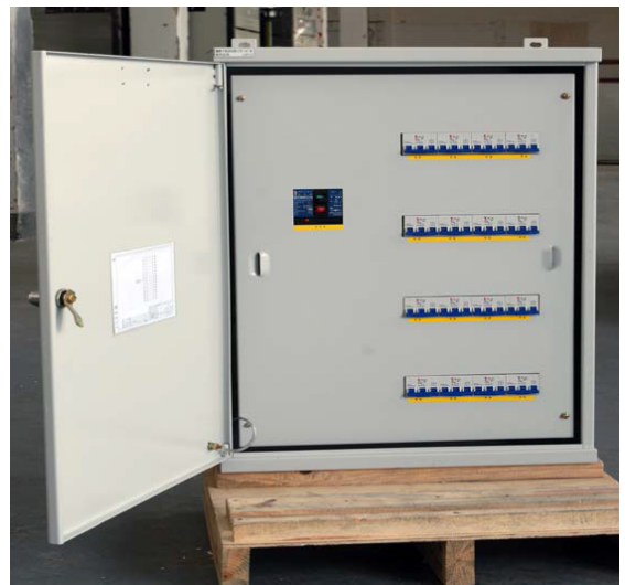
ATS distribution equipment
